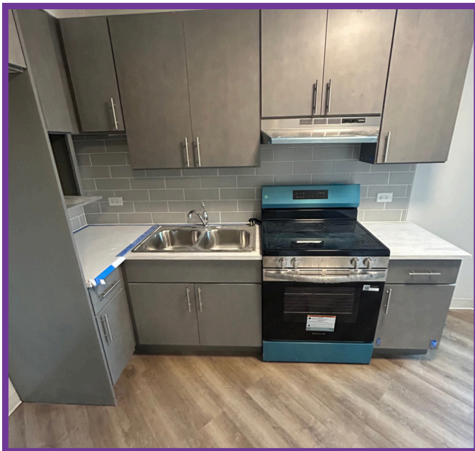
*Blue area on stove is a protective layer that will be removed prior residents returning
